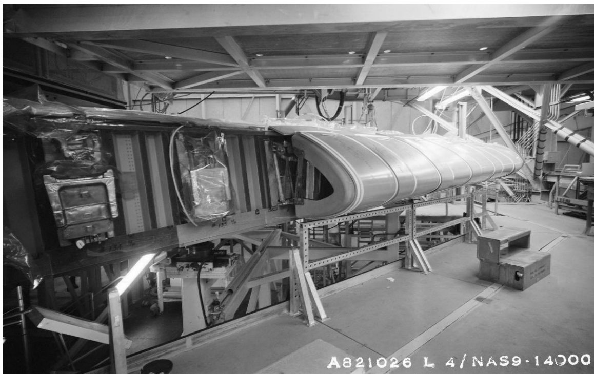
Figure B-31. Installation of wing leading edge on Discovery's port wing in High Bay 2, AFP 42, October 26, 1982.
