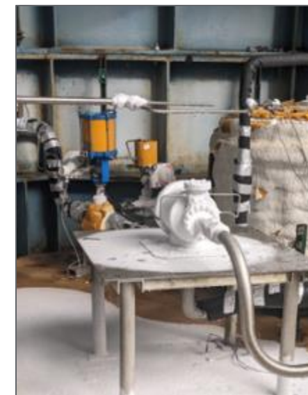
Low-leakage relief valve during LH2 testing
