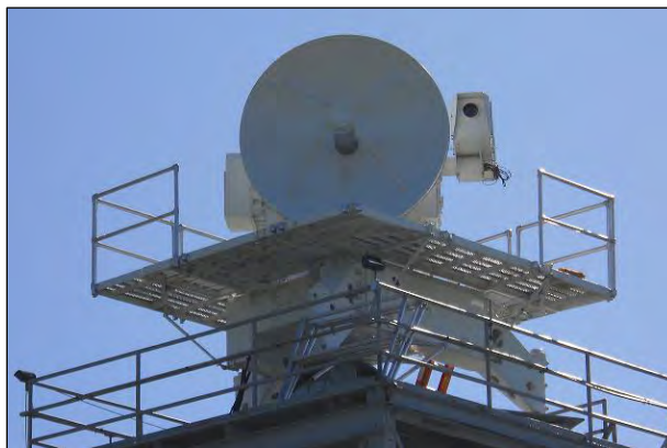
Figure 2–46. Tripod-Type Mobile Radar (shown on an elevated platform)
