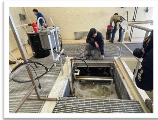
Aeration Basin at Wallops Wastewater Treatment Plant (WWTP)
