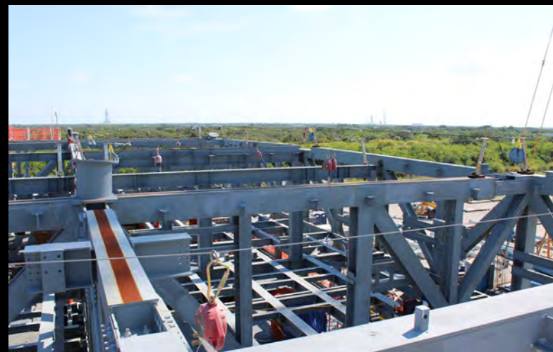
Progress on the ML2 base build-out as seen from above as of August 20, 2024
