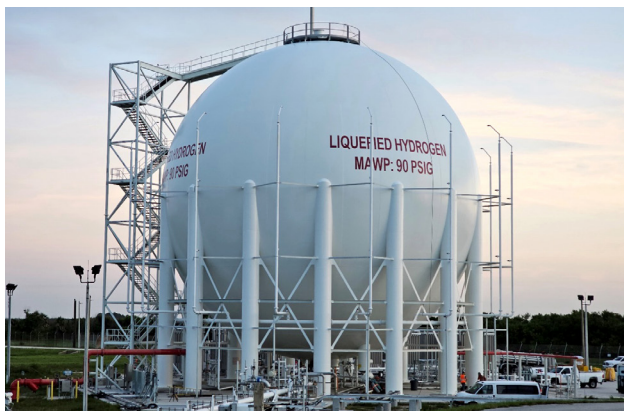
Figure 1: The new 1.3-million-gallon LH2 tank.
