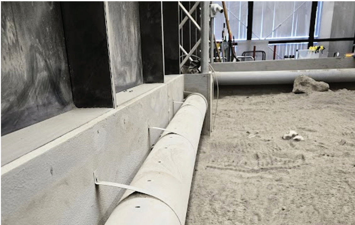
Figure 1: Beacon Mounting locations (note: the ducts along the sides of the Arena walls are 17cm diameter).
