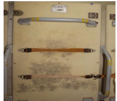
Fungal contamination on ISS panels caused by hygiene activities
