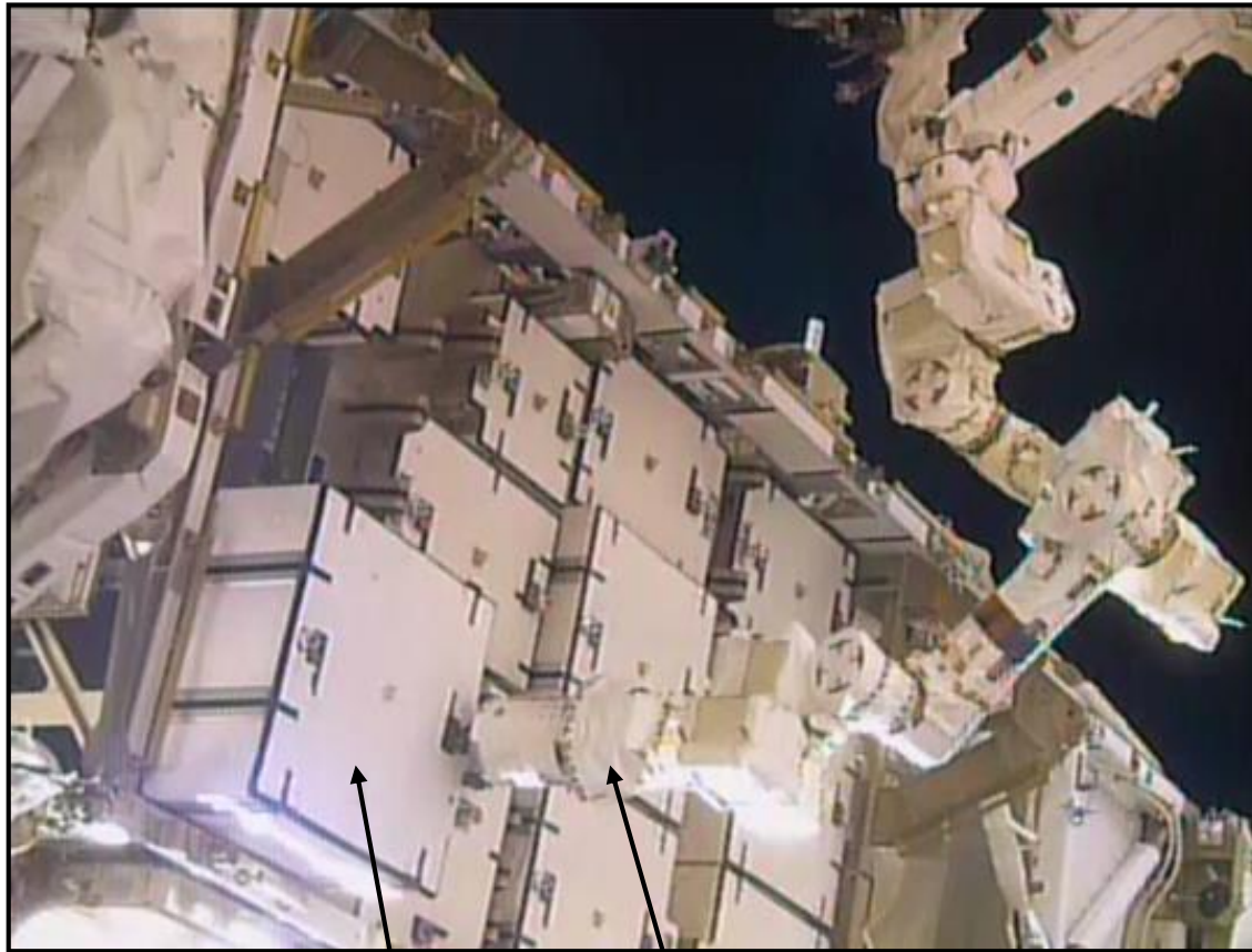
Li-Ion Battery ORU
