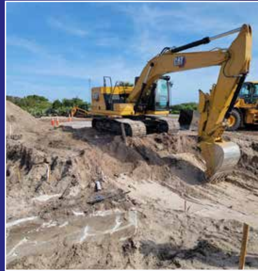
Cleanup crews use all kinds of equipment, including large construction machinery, to remove contaminated soils at Kennedy Space Center. Photo credit: HydroGeoLogic/Dustin Lupis
