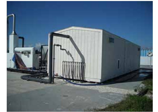
This building houses the hydraulic containment and air sparge system used for treating volatile organic compounds at historic Launch Complex 34. Photo credit: Tetra Tech/Dan Forester
