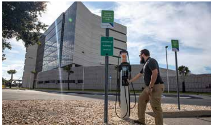
These electric vehicle charging stations at Kennedy's Central Campus Headquarters enhance the spaceport's electric vehicle charging capability while providing employees opportunity to pay for charge-ups of their personal vehicles while they work. Photo credit: NASA/Kim Shiflett
