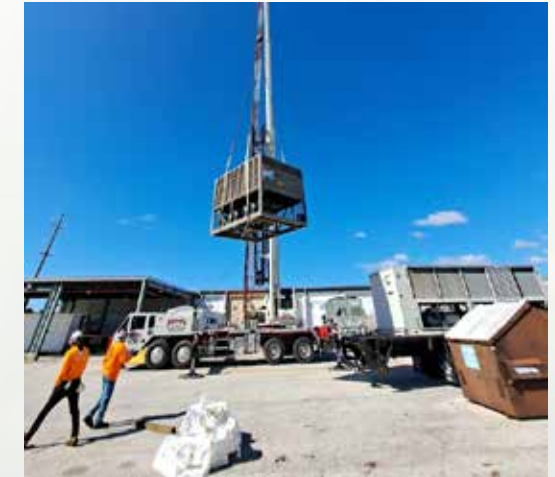
Construction workers off-load new equipment for installation as part of Kennedy's efforts to save money and create a more efficient, resilient and secure energy grid. Photo credit: NASA/Manuel Docurru
