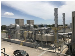
CHP at Building 24
