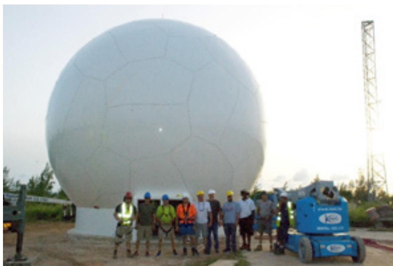
Telemetry antenna in its new protective radome.
