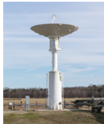
The newly installed 6-meter medium gain antenna system.
