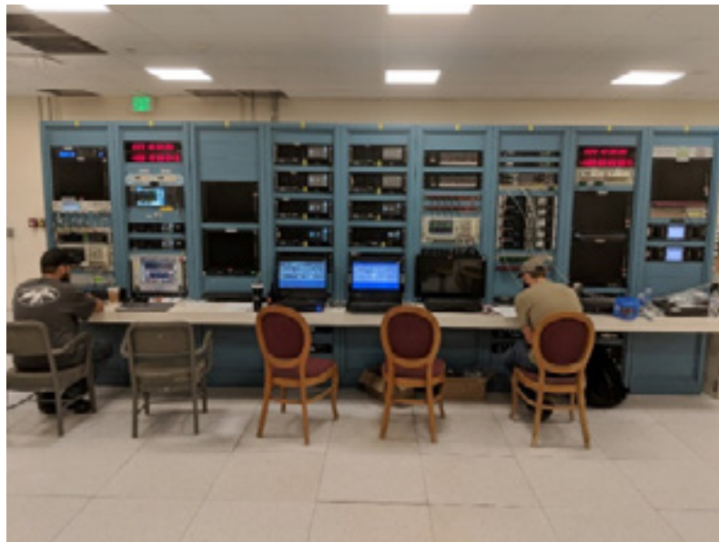
Telemetry receiving and control systems in the Bermuda operations center.
