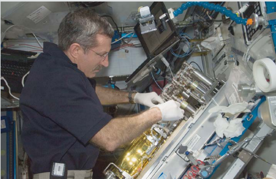
At a workstation in the ISS Harmony node, astronaut Dan Burbank replaces a catalytic reactor in the water recovery system.
