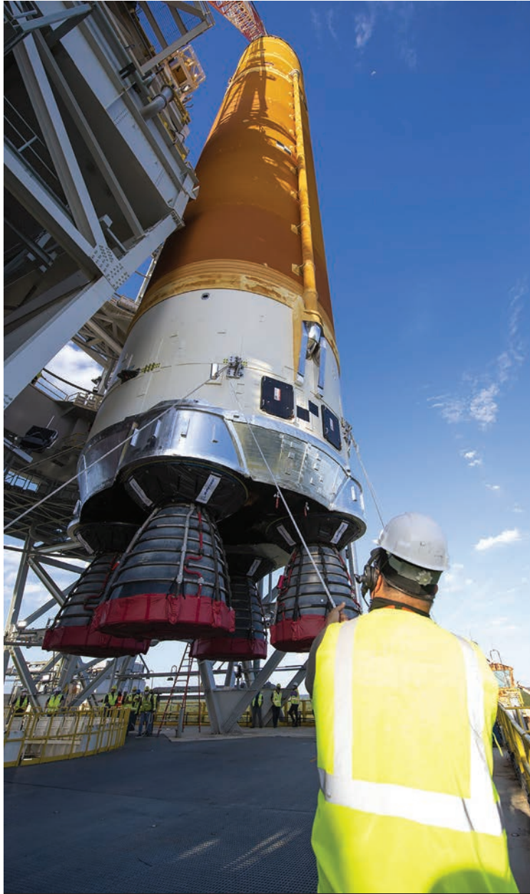
Crews at Stennis Space Center worked to remove the core stage from the B-2 test stand April 19-20.
