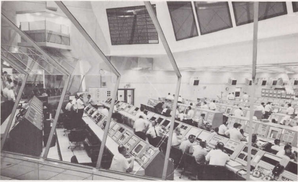
Fig. 147. A firing room in the launch control center; testing of AS-501 is in progress.
