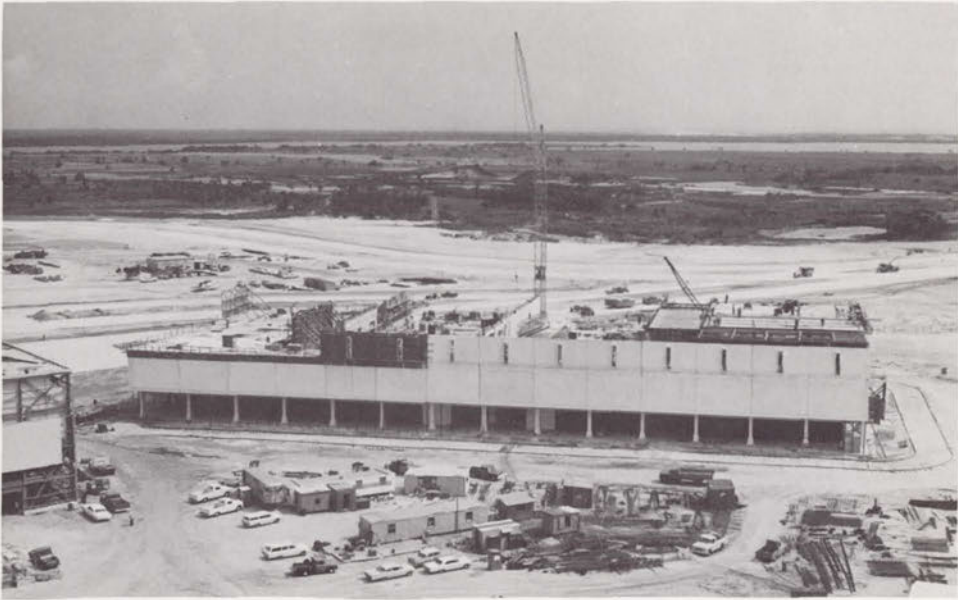
Fig. 77. The launch control center under construction, September 1964. The assembly building shows to the left.
