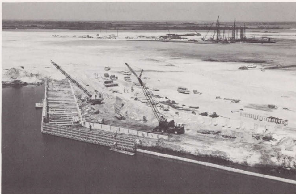
Fig. 68. The wharf under construction at the turning basin, with assembly building site in background, August 1963.
