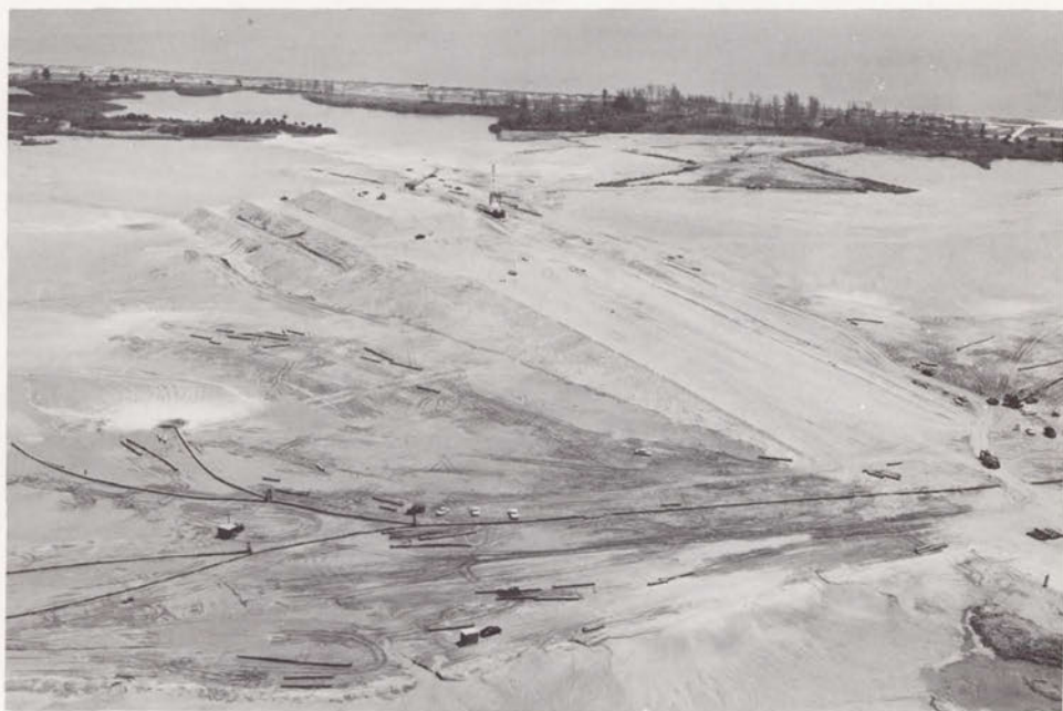
Fig. 69. One of the big sandpiles: hydraulic fill piled on the site of LC-39, pad A, June 1963.
