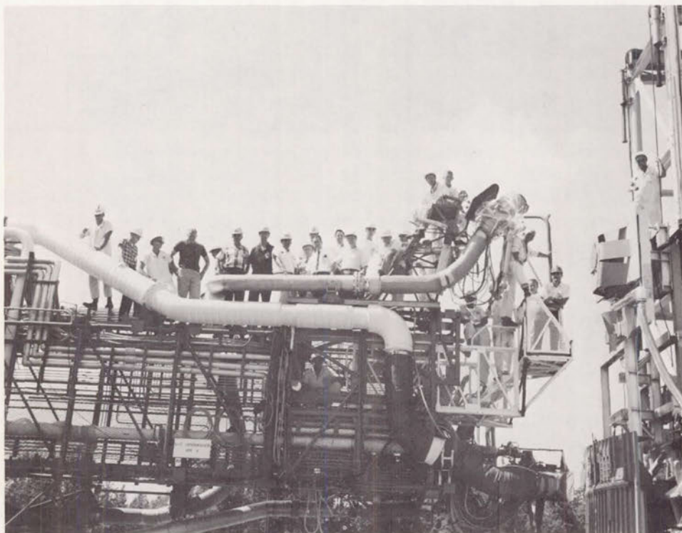
Fig. 94. One of the nine swing (service) arms; when installed, this one would connect to the second stage 43 meters above the base of the rocket.
