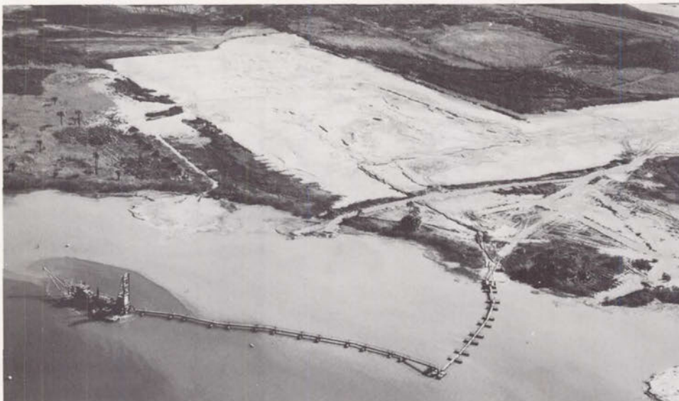
Fig. 66. Dredging hydraulic fill from the Banana River and pumping it onto a construction site, December 1962. The water is draining back into the river above and right of the barge.
