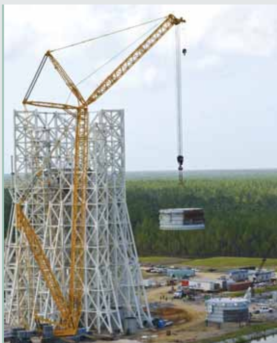
A section of the test cell is lifted for installation on the A-3 test stand's structural steel frame. Work on the A-3 Test Stand began in 2007. It is scheduled for activation in 2012.
