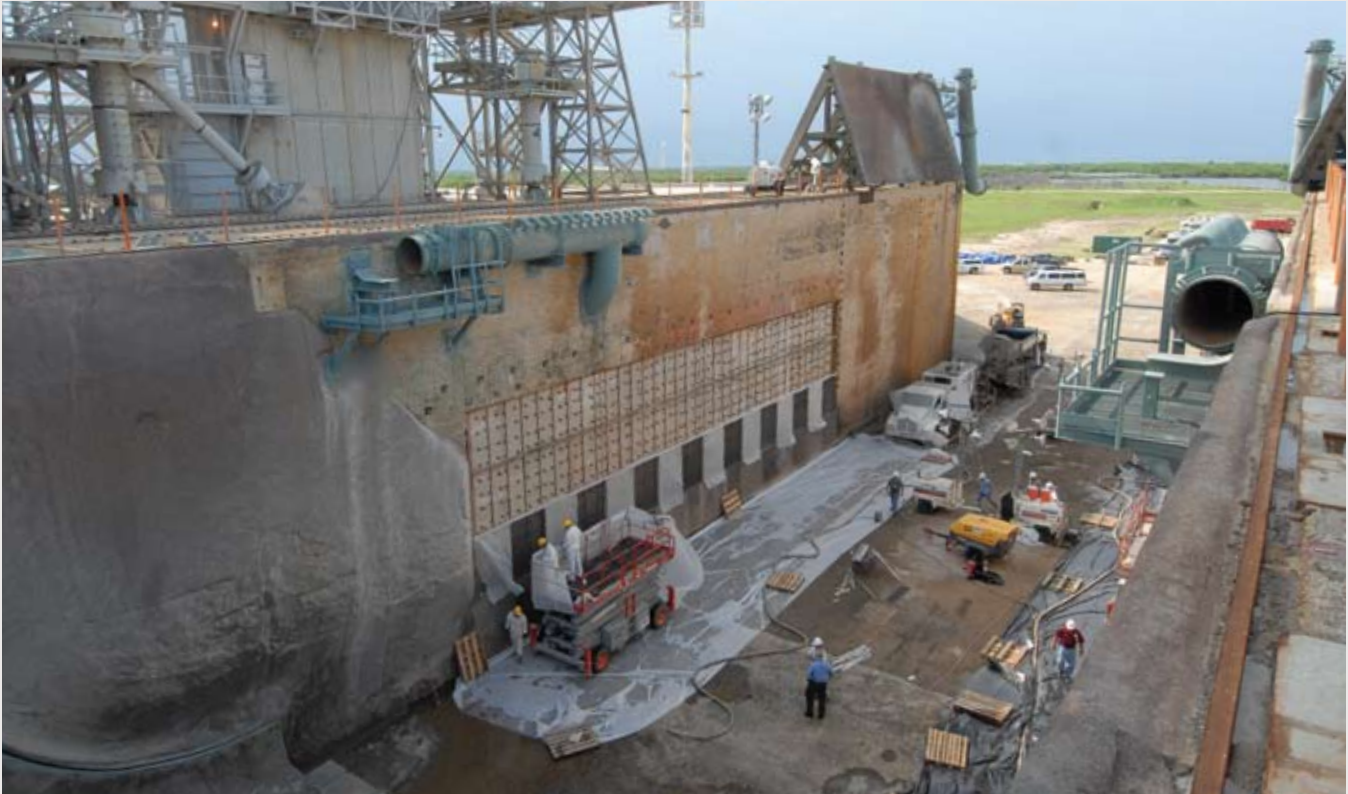
KSC workers repair east wall of Launch Pad 39-A damaged by STS-124 SRB ignition.
