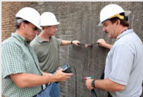
KSC inspectors test repairs on the Fondue Fyre refractory concrete system on the flame trench walls. Fondue Fyre was developed during Apollo.
