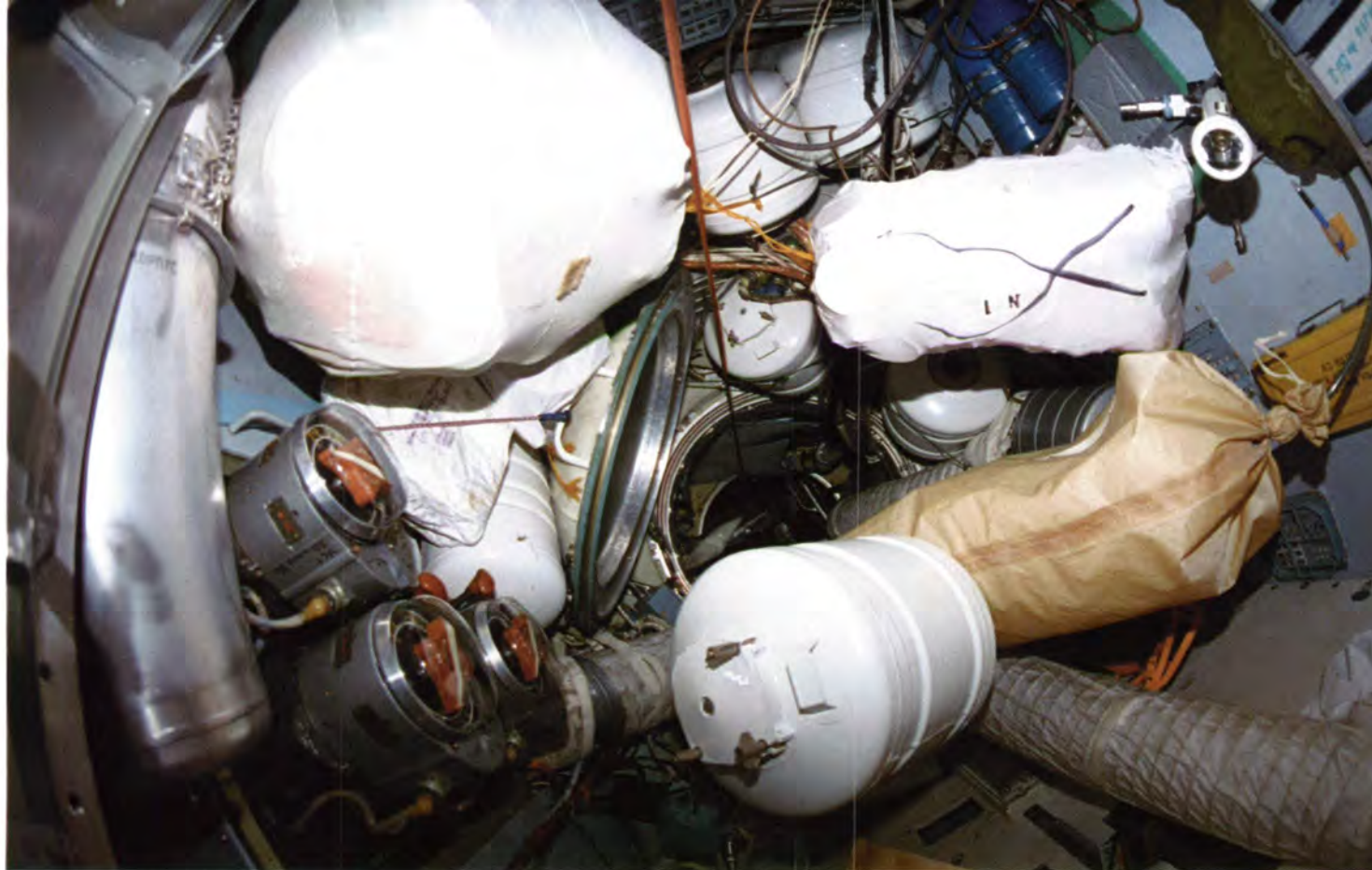
Mir's master alarm sounded on February 24, 1997, to alert the six inhabitants that a fire was onboard. In case of evacuation, crewmembers would have quickly moved through crowded passage-ways (photo left) to escape on the Soyuz. However, crewmembers contained the fire in the Base Block, but not before dense smoke spread throughout the complex. Damage included melted insulation on cables in the Kvant-1 module and charred panels (photos bottom right).
