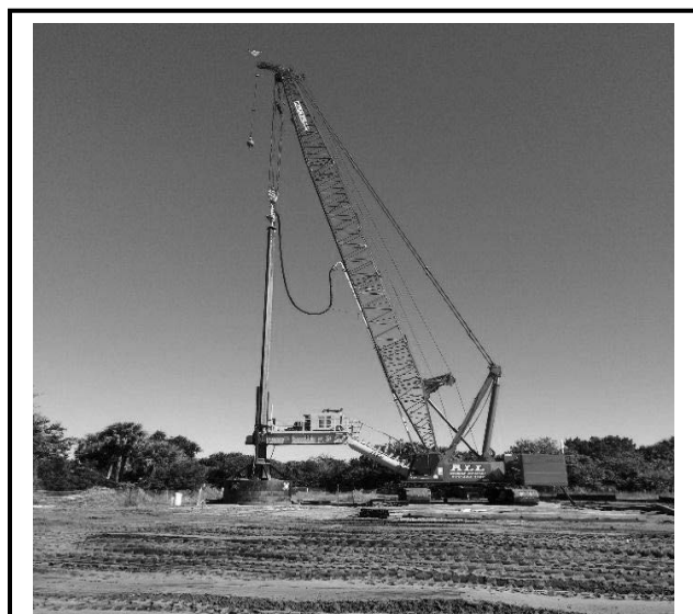
Large Diameter Auger soil mixing with thermal treatment and iron at KSC to remove Chlorinated Volatile Organic Compounds. Crane with a containment shroud shown.
