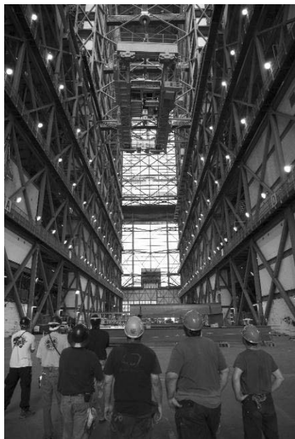
Inside the Vehicle Assembly Building at Kennedy Space Center, the construction crew watches a 175-ton crane lowered from Level 16 to the transfer aisle floor. The Exploration Ground Systems project will upgrade the crane's 45-year-old controls to improve reliability, precision and safety. When upgrades are complete, the crane will provide lift capability for NASA and other exploration vehicles, including the Agency's Space Launch System and Orion crew vehicle.
