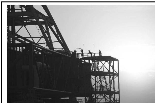
Crews at Kennedy Space Center perform modifications to the Mobile Launcher to accommodate the weight, size, and thrust of NASA's new Space Launch System and Orion crew vehicle. The upgraded launcher will carry the stacked rocket and crew vehicle to Launch Pad 39B for Exploration Mission-1 later this decade.
