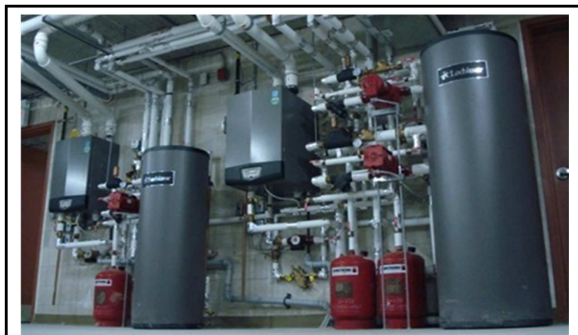
The MSFC Steam Distribution System is the second of a two phase project to convert buildings to a more efficient natural gas fired boiler system that reduces operating and maintenance costs.
