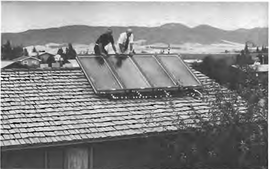
In the energy-conscious era of the 1970s, NASA's operational experience found many new applications. This prototype water heater, warmed by solar cells, was installed on a home in Idaho.
