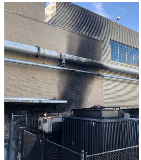
A transformer fire at GRC, caused by degraded electrical equipment, must be repaired to sustain mission work
