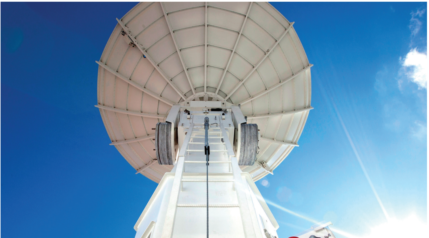
Part of the Kennedy Uplink Station, the S-band ground tracking system at Kennedy provides crucial tracking and communication capabilities following liftoff of SLS and Orion.
