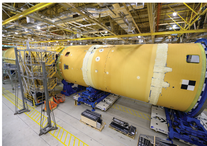
Connecting feedlines and other external components to the fully assembled Artemis I core stage at Michoud.
