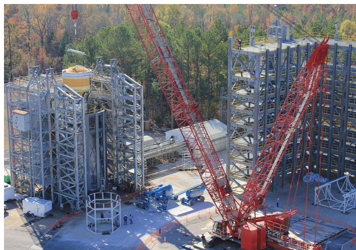
The Integrated Structural Test at Marshall included applying loads 40 percent greater than expected during launch to test versions of the launch vehicle stage adapter, frangible joint assembly, ICPS, Orion stage adapter, and a mass simulator for Orion.
