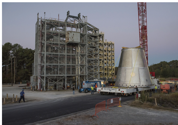
The launch vehicle stage adapter structural test article for the Integrated Structural Test was manufactured and tested at Marshall.
