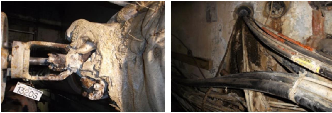
Figure 2: High Pressure Lines in a Langley Research Center Utility Corridor
