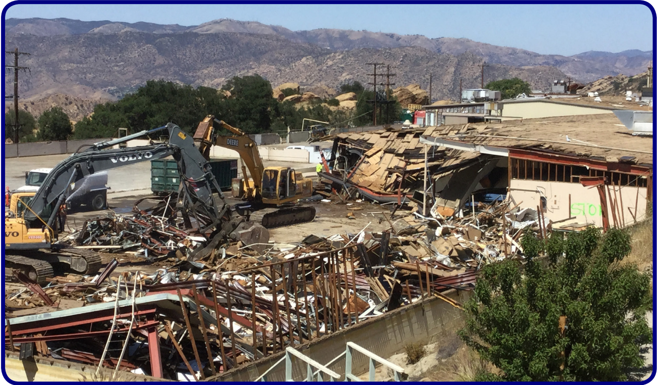
Image Caption: Buildings are demolished at NASA's Santa Susana Field Laboratory in California. (Credit: NASA)
