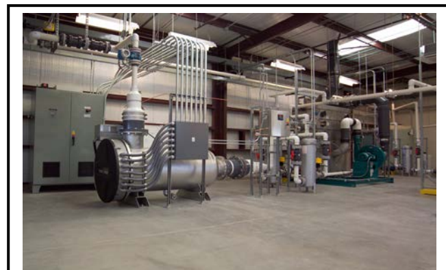
The Mid-Plume treatment system at WSTF (pictured here) uses an ultraviolet (UV) reactor to treat the N-nitrosodimethylamine (NDMA) contaminated groundwater. Ultraviolet lamps disperse UV light into the water, breaking the chemical into harmless byproducts. To support Sustainable Remediation, the UV reactor is powered by an onsite photovoltaic system.
