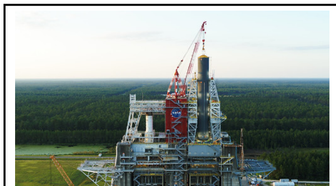
NASA's Space Launch System (SLS) core stage pathfinder, shown here, is positioned in the B-2 Test Stand at NASA's Stennis Space Center (SSC) near Bay St. Louis, Mississippi. SSC work crews used it in August to train and practice handling and lifting techniques needed for the core stage flight hardware when it arrives at SSC for testing in 2020. These efforts will enable a successful Moon landing in 2024.
