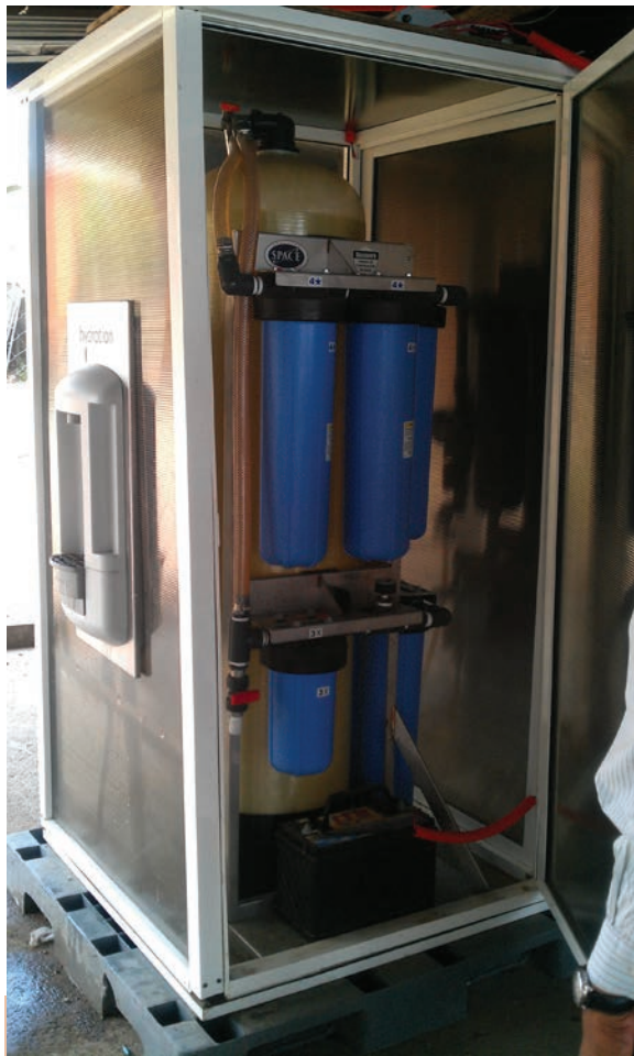
Filtration system providing clean, safe water installed at a school in Chiapas, Mexico.
