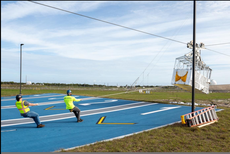
January 24, 2024—In preparation for the Artemis II crewed mission, EGS teams begin installation of four emergency egress baskets at Launch Complex 39B
