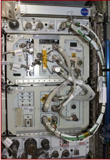
Figure 4.3.1. Picture of DECLIC for the Study of Critical Liquids and Crystallization. (Source: Centre National d'Etudes Spatiales/NASA)
