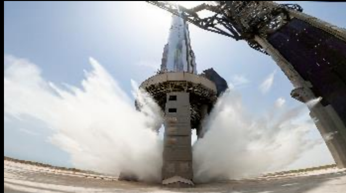
July 28, 2023 — Full pressure test of the newly installed Starship flame deflector, part of the redesigned orbital pad at SpaceX's Starbase in Boca Chica, Texas.
