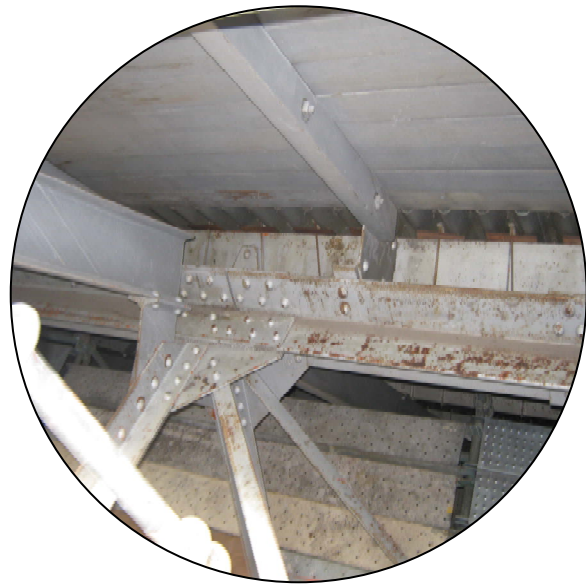
Figure 3-14: Corrosion at Gabled Frame Framing Below Window.
