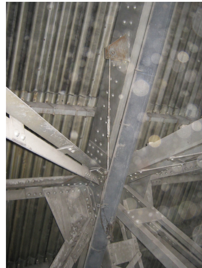
Figure 3-26: Typical Pipe Support at Hangar Wall
