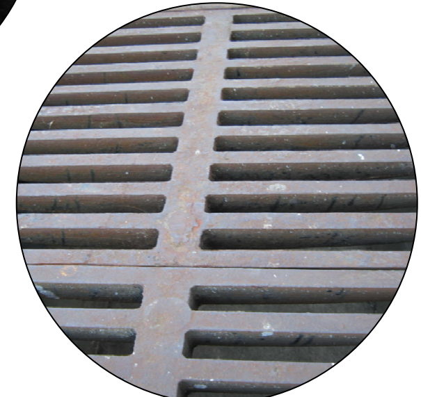
Figure 3-30: Typical Original Grating
