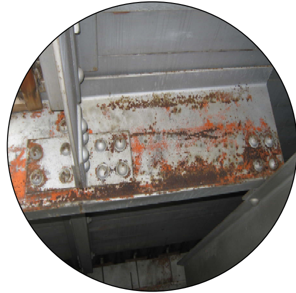
Figure 3-15: Corrosion at Wind Girt Below Window
